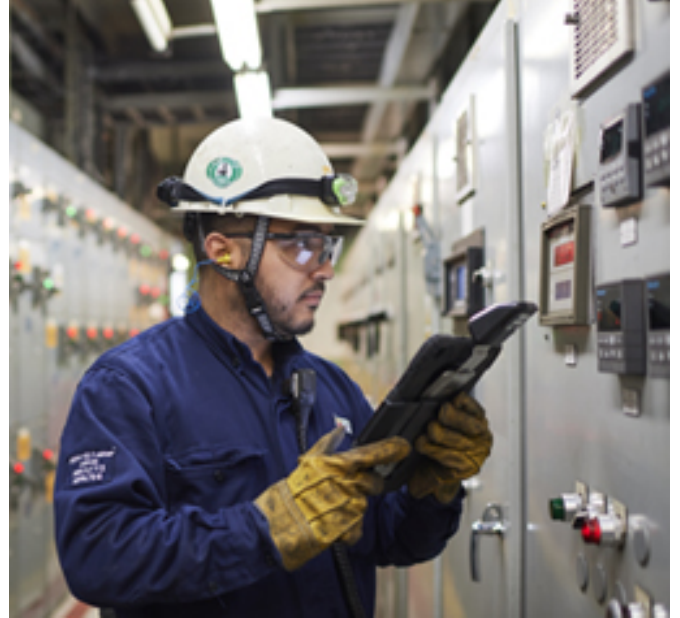
Implementation of mobile monitoring capabilities. Efficient, real-time analysis of equipment parameters during maintenance inspections.
