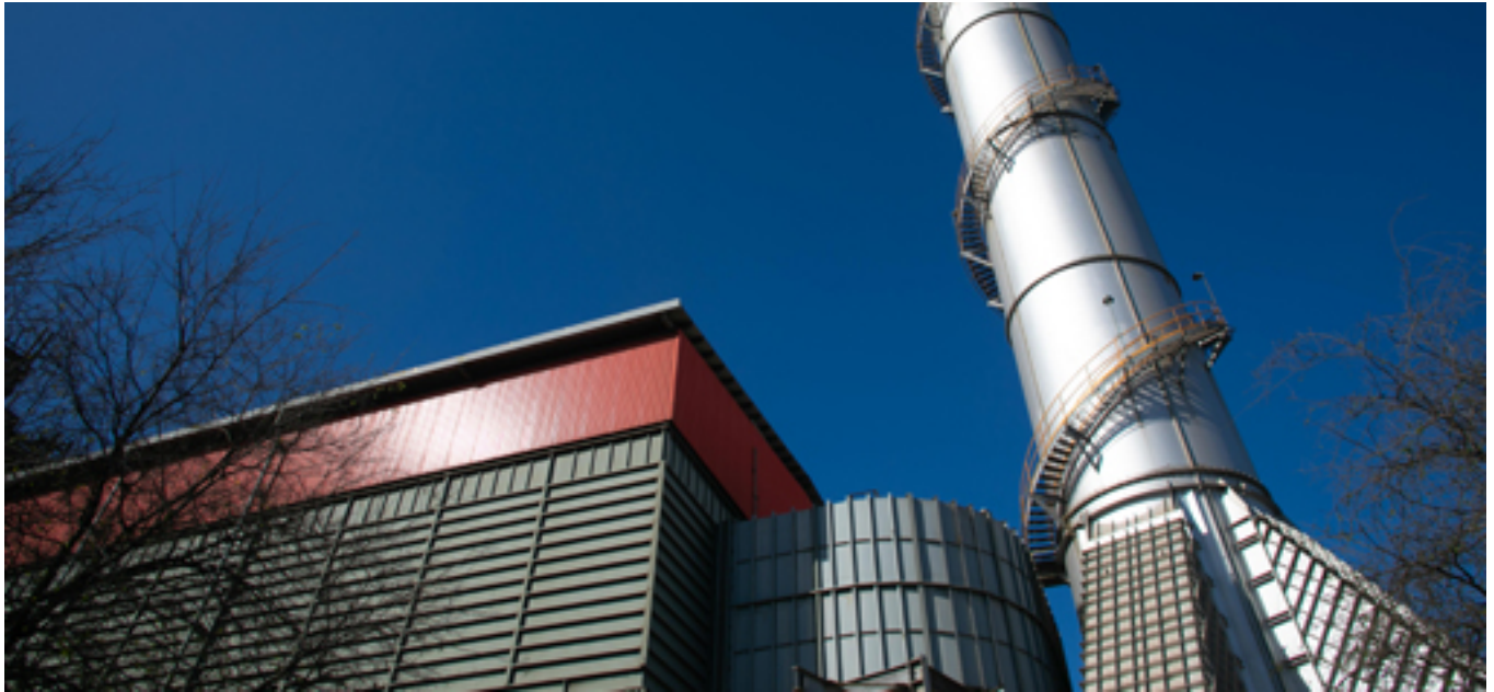
Adopting the best-available technologies. In the last five years, Ternium has made investments of approximately $137 million to improve the capture and treatment of air emissions.
